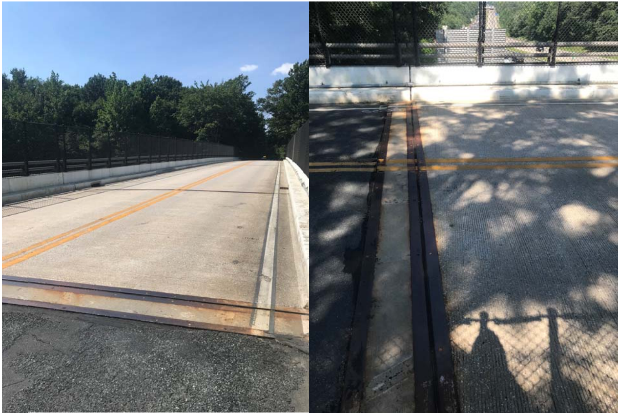
Photos of CEX95200 taken by the BEST Center during field visit (Girders, bearing condition and substructures cannot reach)
