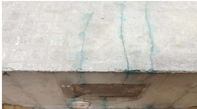
Figure 2 - Fine cracks identification
