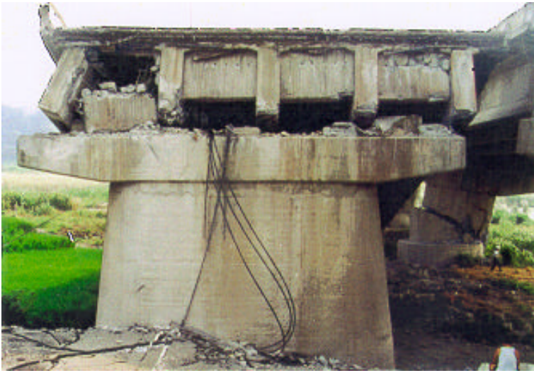
Figure 9 - Crushed End Diaphragms and Shear Blocks at Pier P1N
