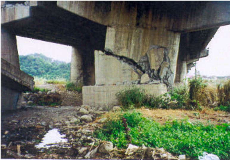
Figure 8 - Shear Cracks on the Southbound Hammerhead Concrete Pier p2S
