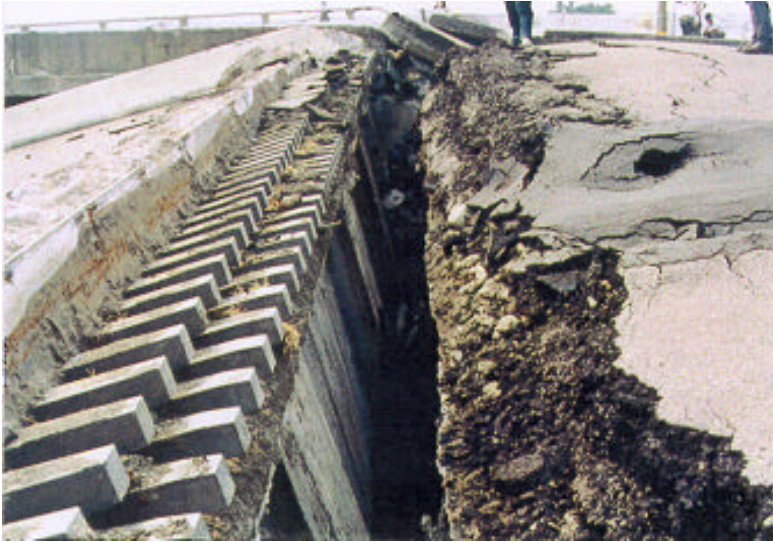
Figure 7 - Backfill Upward Movement at the North Abutment of the Northbound Bridge
