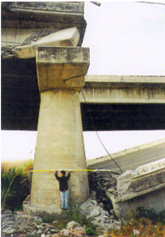
Figure 6 - Fallen Beam due to Superstructure Movement in the Longitudinal Direction at Pier P2N
