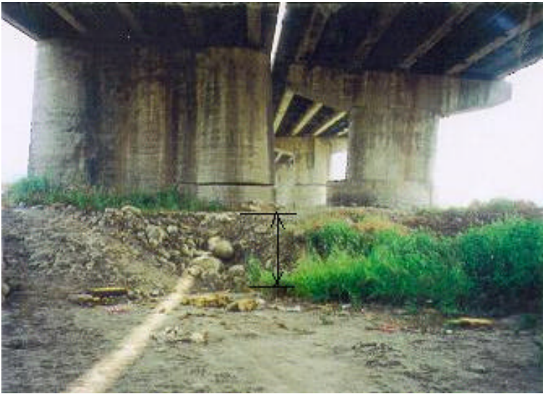
Figure 5 - Oblique Fault Movement between Piers P3N and P3S
